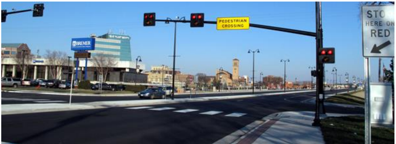
Figure 3-15. High-Intensity Activated Crosswalk Beacon (HAWK) or Pedestrian Hybrid Beacon (PHB)
