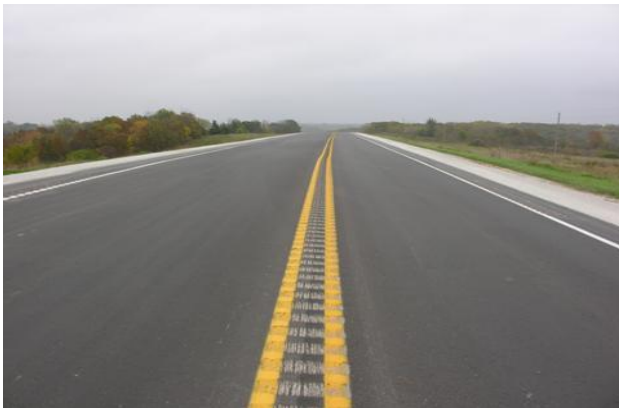
Centerline Rumble Strips
